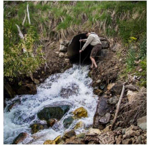
Tributary culvert that dozens of PIT-tagged fluvial cutthroat trout have ascended during spring spawning.
