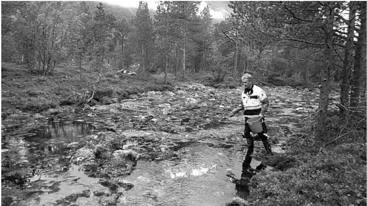
FIGURE SOP 13.4. CatSan Hygiene Litter/CFT Legumine mixture granules being spread by hand to upwelling groundwater area.
