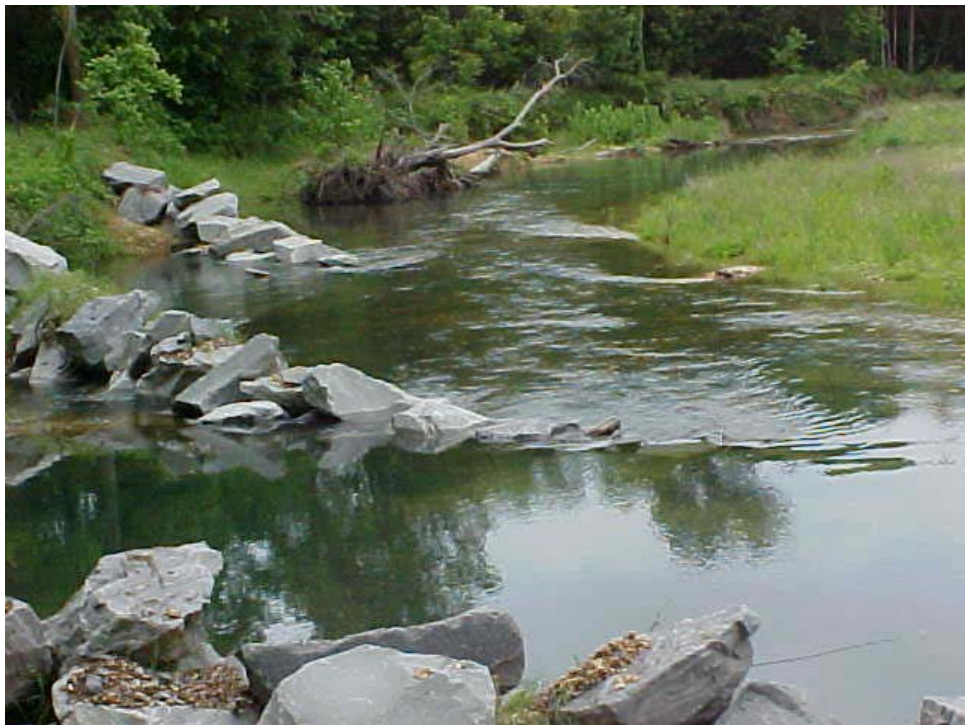
Figure 2. Picture of J-hook rock vanes installed at Spring Creek in northeast Oklahoma.
