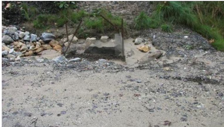
Failed sediment screen on a road cross drain inlet in the brook trout stream watershed, September 2009.
