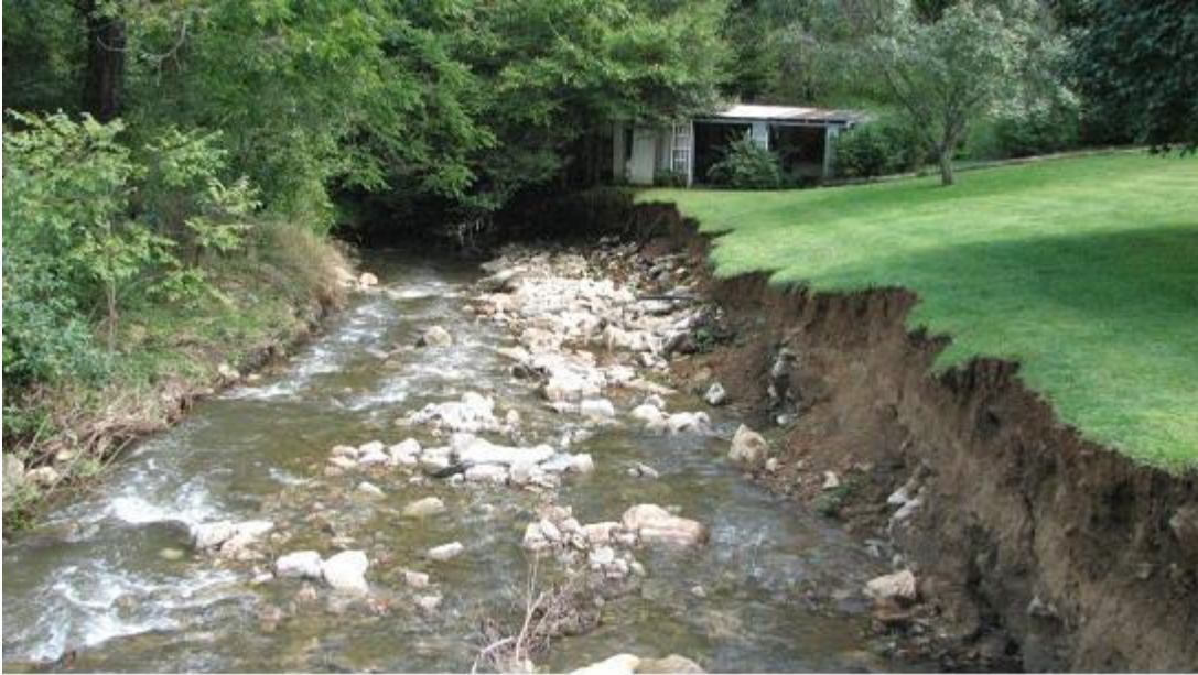
2010 flood damage in northwestern Yancey County
