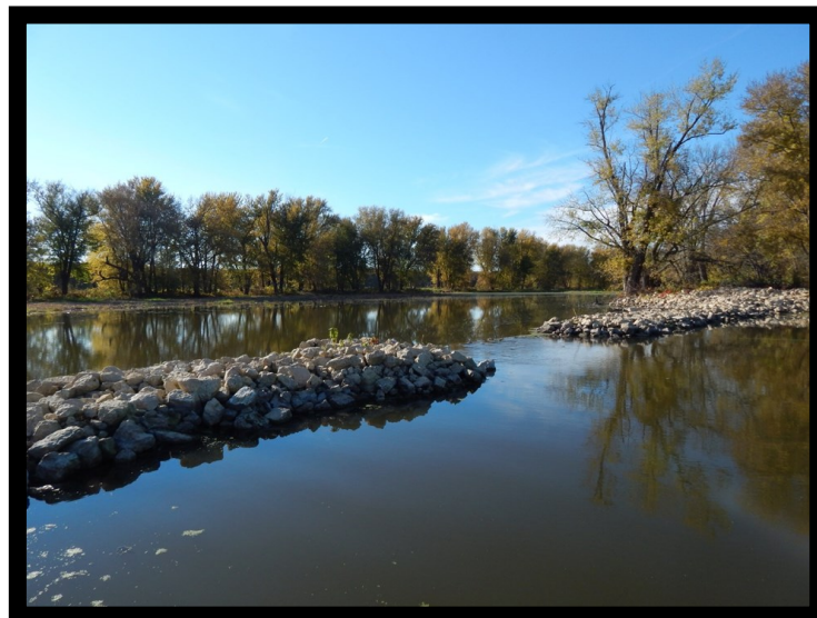
Figure 2. Rock closing structure designed to reduce flow and sediment delivery into Sunfish Lake.
