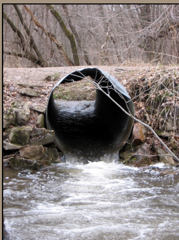
Road culvert on a small stream in rural Wisconsin, USA. Photo credit: Carmen Hardin, Wisconsin Department of Natural Resources
