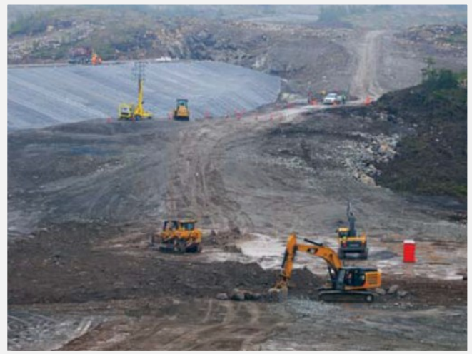
Sandy Pond being converted into a reservoir for toxic waste (Vale newsletter)
