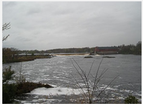
Great Works Dam on the Penobscot River shortly before removal began in June 2012. Photo credit: Shelley Dawicki, NEFSC/NOAA.
