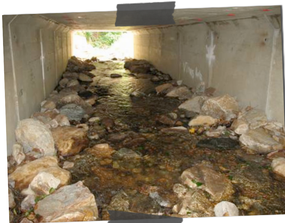
AOP friendly box culvert constructed by the Vermont Transportation Agency in Readsboro, VT.
